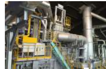
Clervaux remelter investment - improved recycling capabilities
