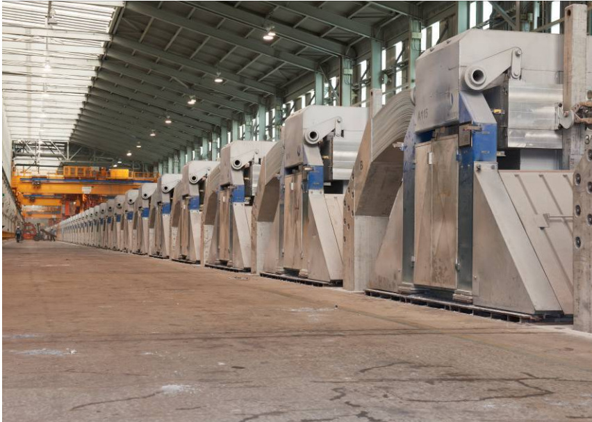
2x1.2 km of electrolysis cells
