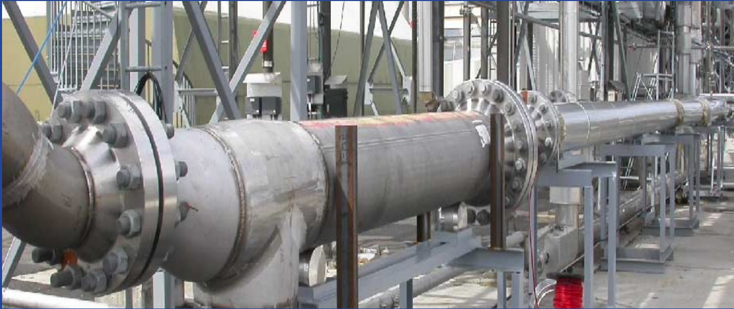
The pipe separator; a new concept for subsea processing
